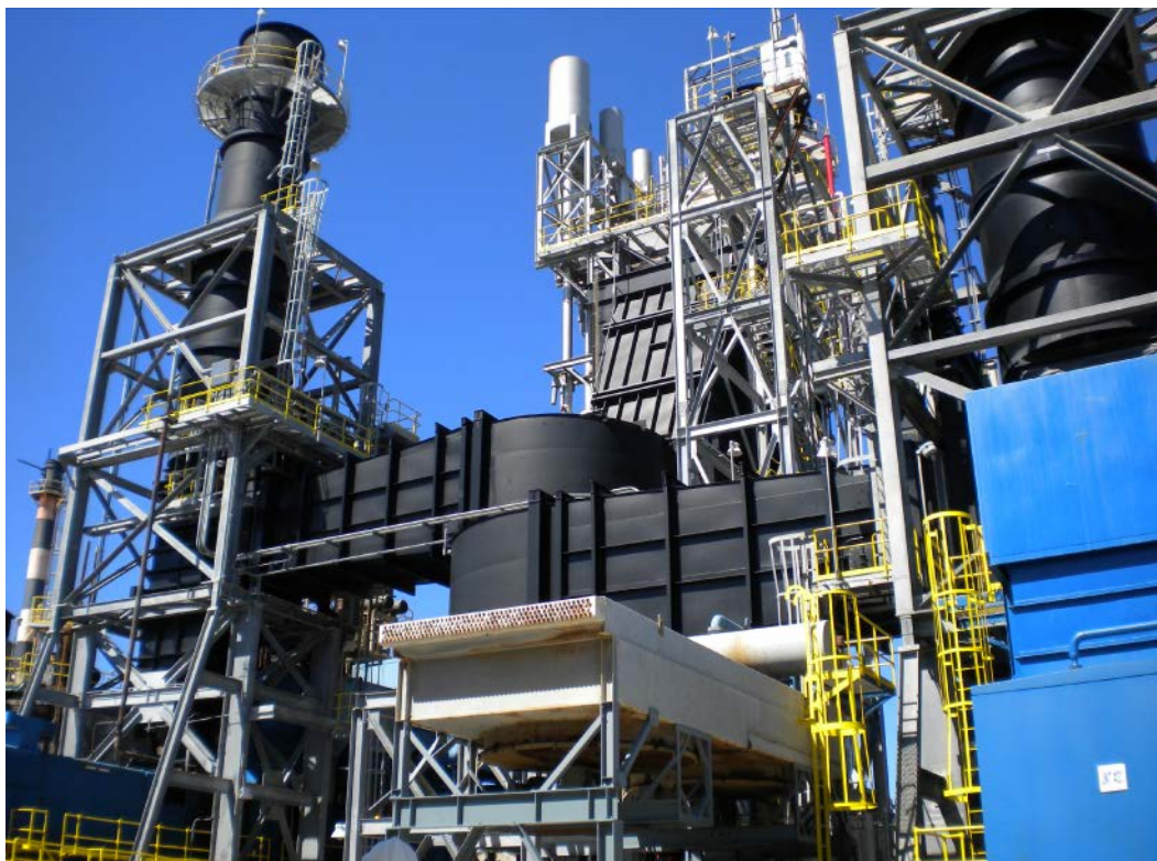
Figure 12. Heat recovery steam generators on St. Croix
